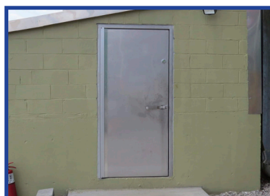
Mechanical Room Flood Door (PD-525)
