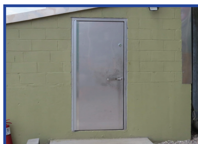
Mechanical Room Flood Door (PD-525)
